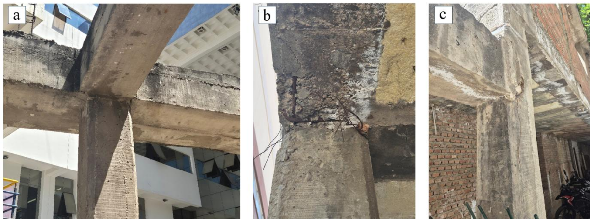
Figure 7. (a) Beam–column joint, (b) reinforcement corrosion, and (c) concrete deterioration.
