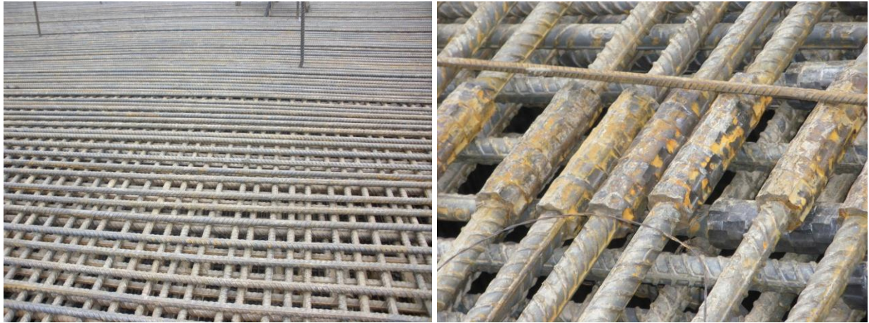
Figure 12. The superior reinforcement consisted in two double layers of 32mm rebars. SCC concrete mix was designed to pass through this reinforcement.
