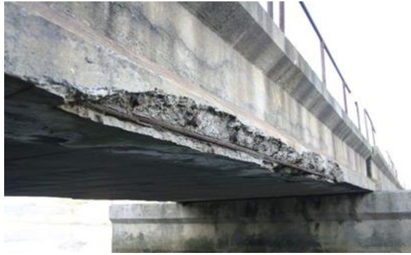
Figure 1. Corrosion-induced damage on a concrete bridge exposed to air-borne chlorides close to the shore in Cape Town
