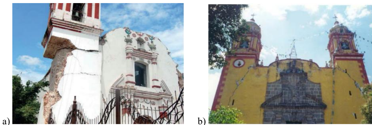
Fig. 1. Trend of deterioration and failure in bell towers attached to adjacent bodies, a) horizontal failure by earthquake with a tendency to tip over at the top by abrupt change in volume. Image taken from of the Ministry of Culture, Government of Mexico (2024), b) diagonal failure by earthquake by abrupt change in section. Image taken from: De la Torre R. O., et. al. (2004).
